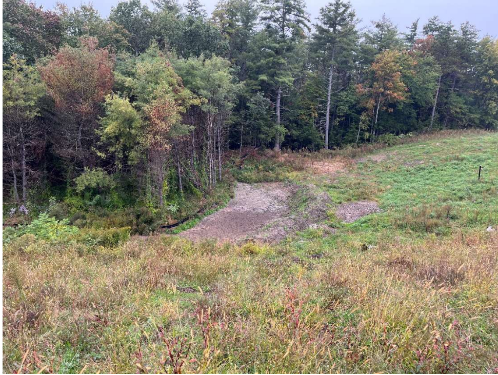
Photo 5 – Southwestern slope with sediment cleared away from the erosion control.
