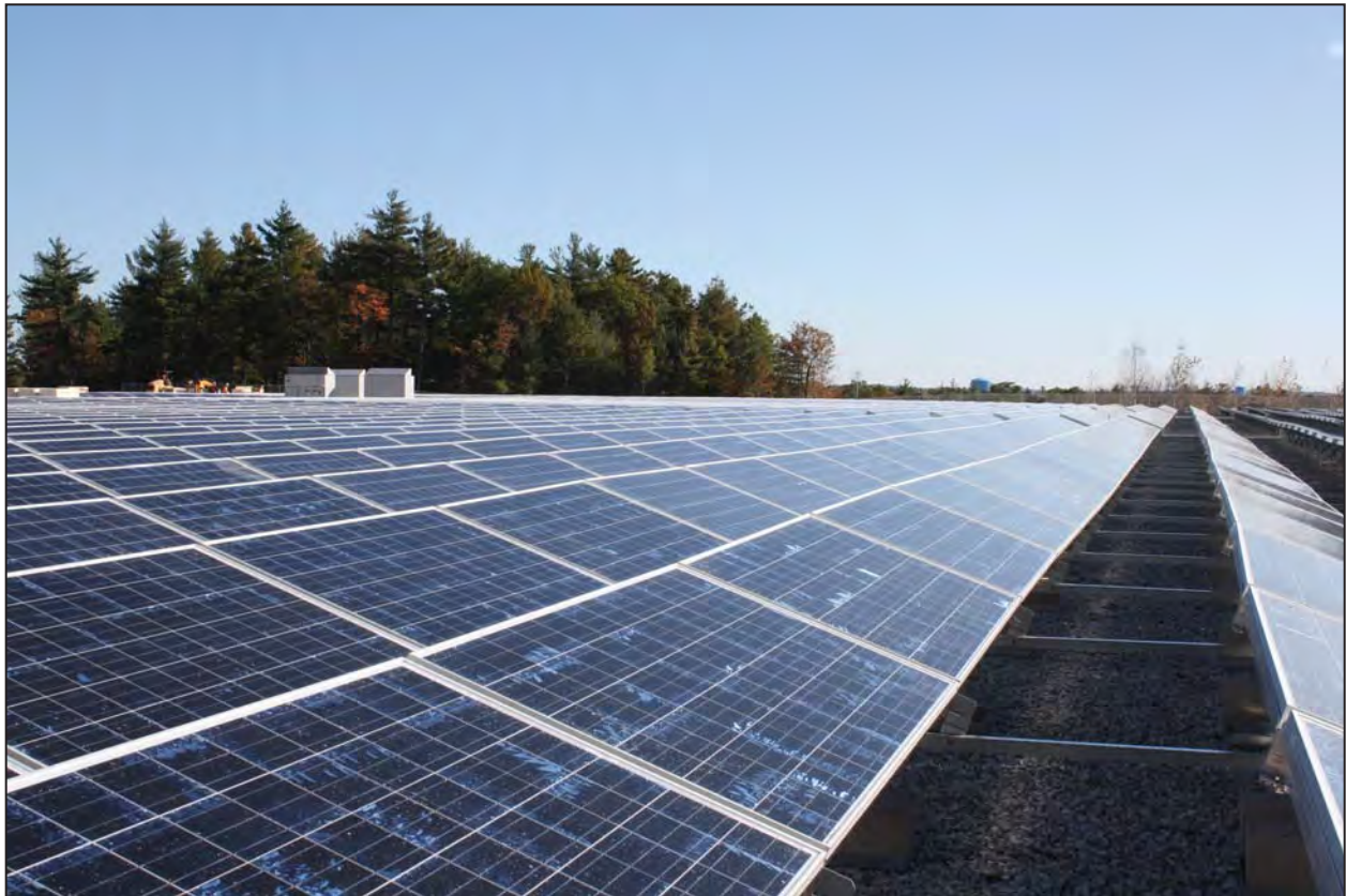
Westford Solar Park, photo courtesy of EEA
