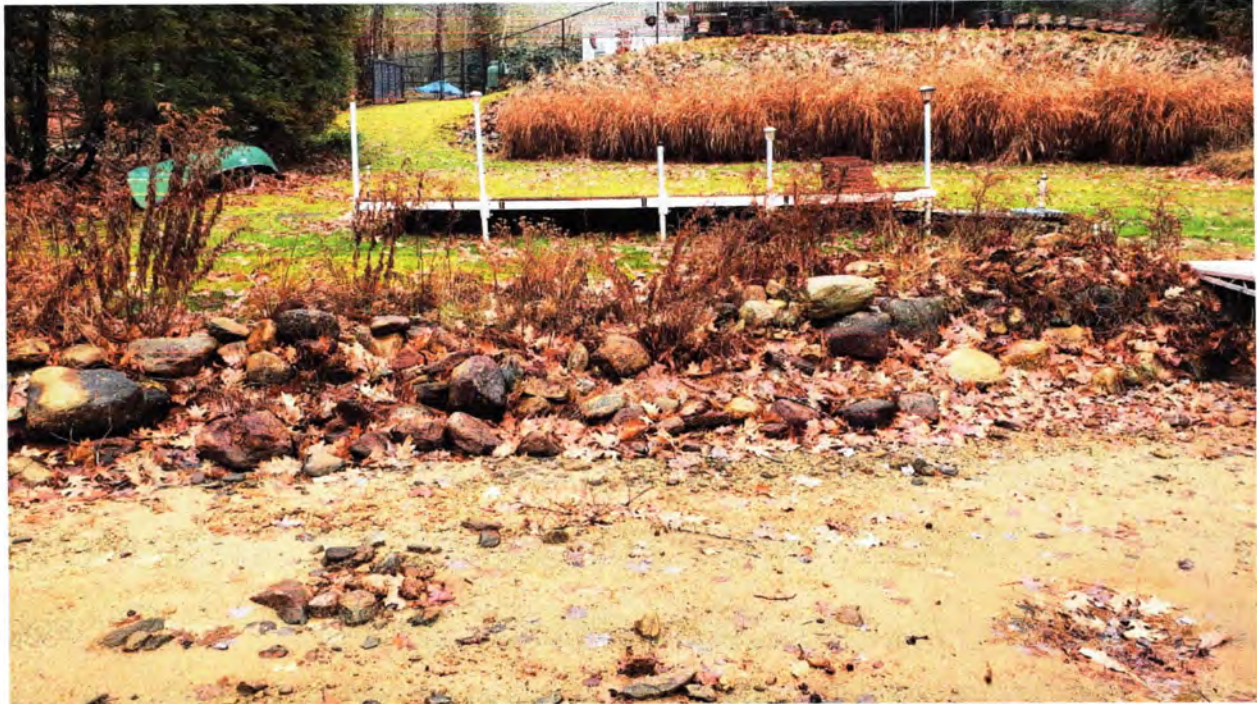
Views of current deteriorating rock wall from the lake
