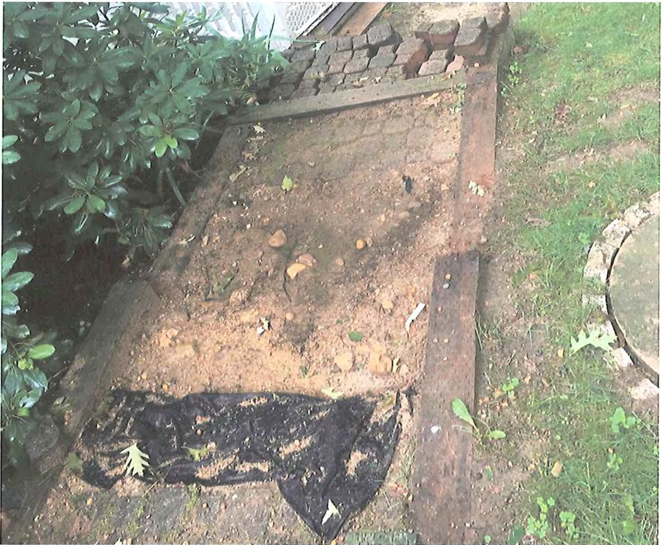
Street side walkway steps needing repair + replacement.
