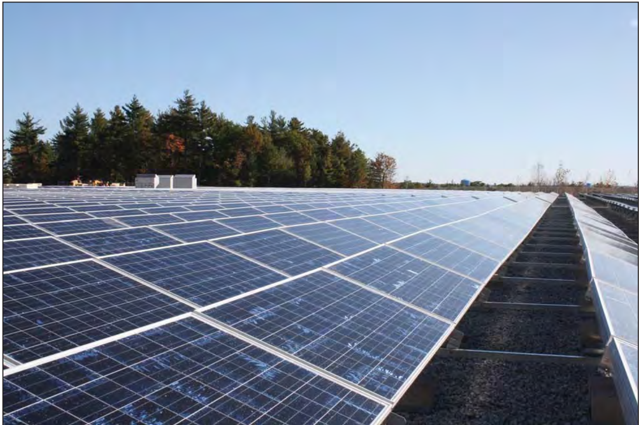
Westford Solar Park, photo courtesy of EEA
