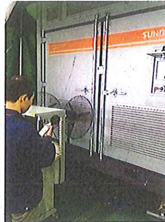
1m away from Inverter
