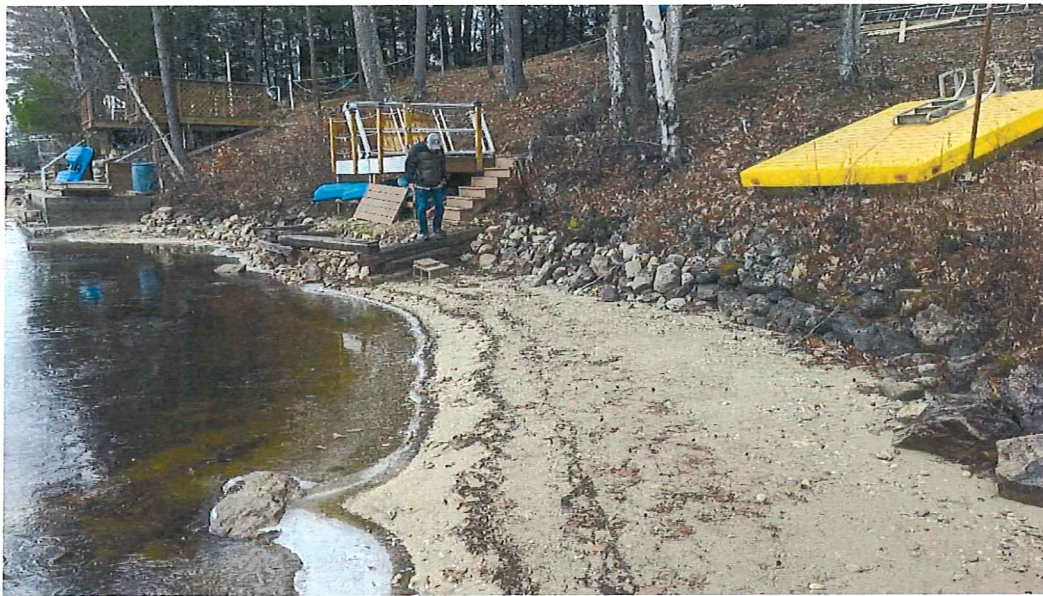
Figure 1. Winter photo of eroded shoreline facing north. Rocks from eroded stone retaining wall have been placed along shoreline to reduce erosion. Lake draw down conditions allow for stone wall to be constructed in the dry.
