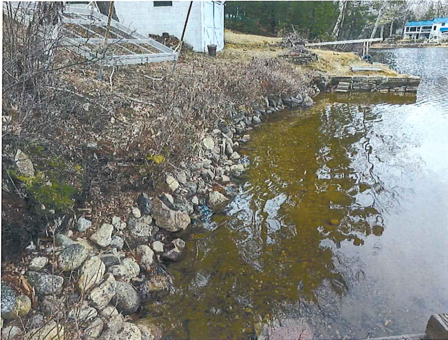
Figure 3. Fall photo facing south from center of shoreline. Shows neighboring concrete wall where restored stone wall will tie into.
