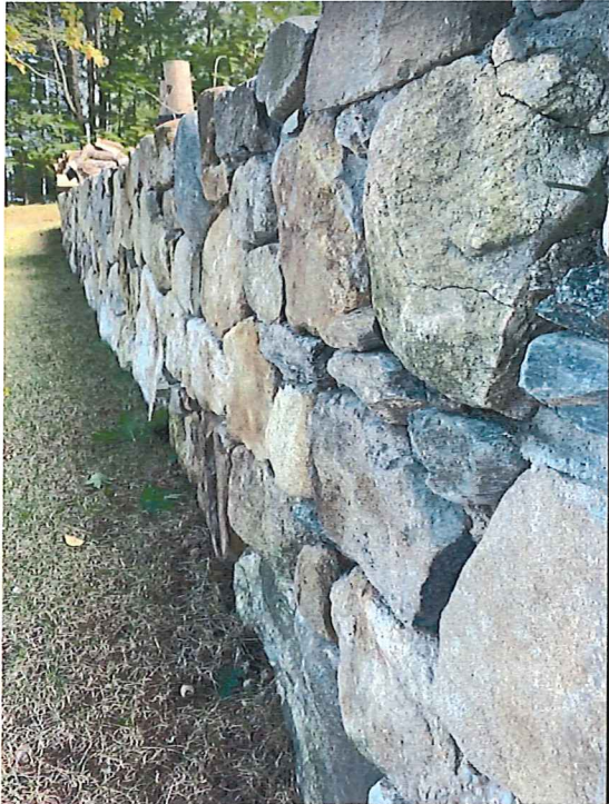
Figure 7. Image of stone wall installed on property above OHW. The same style will be used on the restored stone wall for shoreline stabilization.
