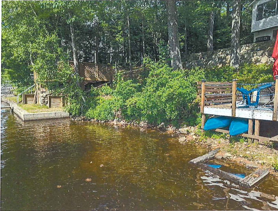
Figure 5. Summer photo showing northern end of shoreline. Railroad ties to be removed.
