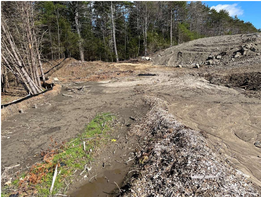
Photo 11 – Silt buildup at southwestern limits of the Site.
