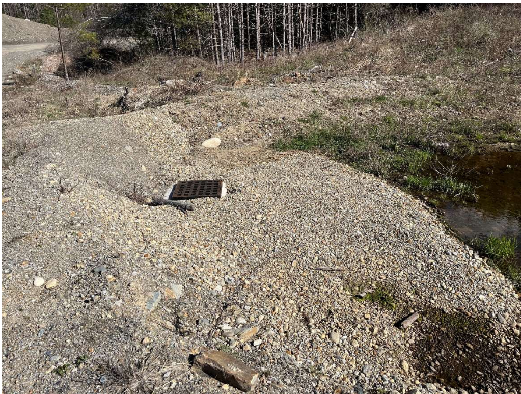
Photo 4 – Temporary stormwater overflow catch basin.
