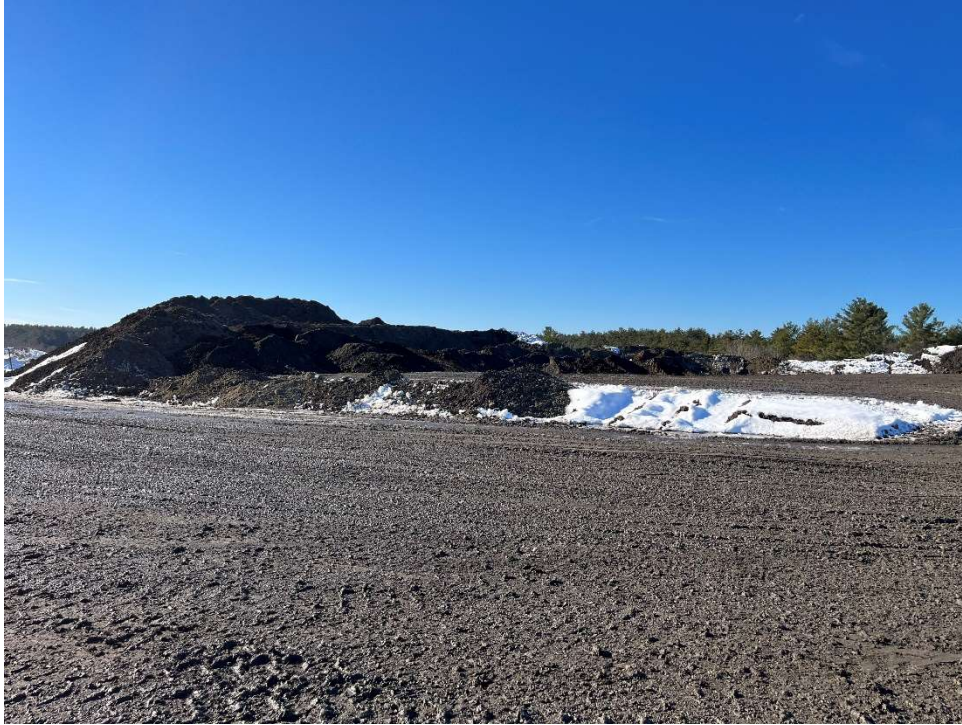
Photo 13 –Material placed and graded at the center of the Site with grading for truck access
