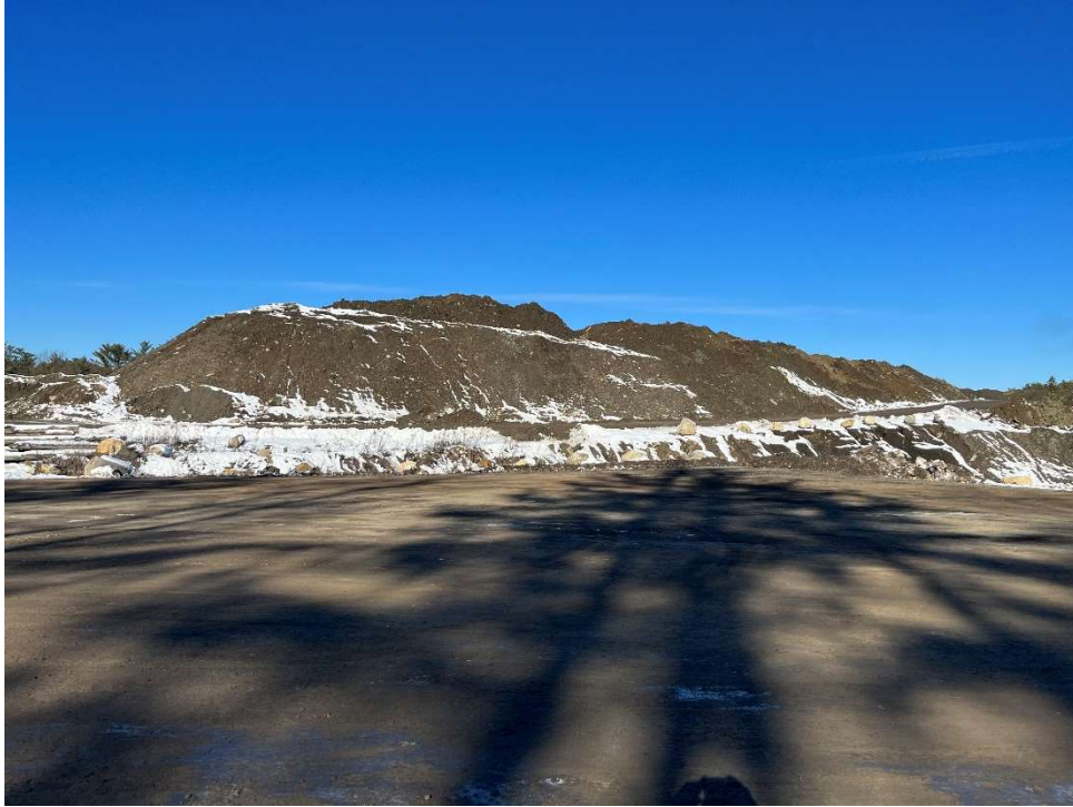
Photo 3 –Material placed and graded at the center of the Site with grading for truck access
