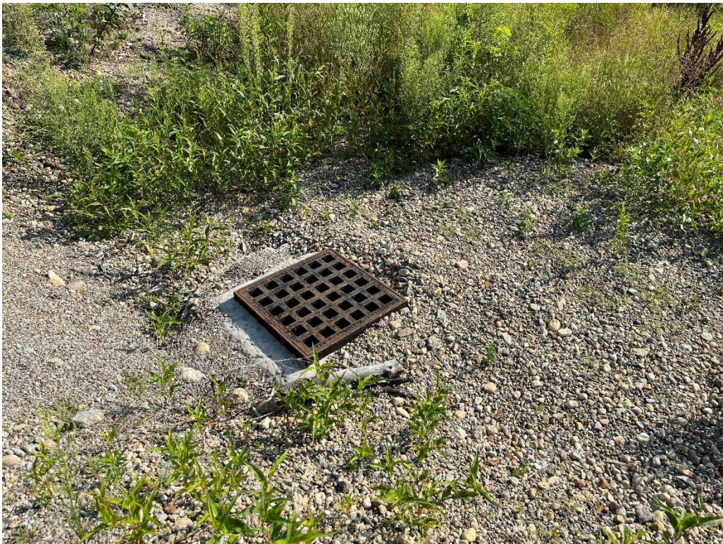
Photo 4 – Temporary stormwater overflow catch basin.
