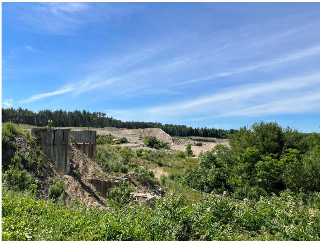
Photo 12 – Existing slope and erosion control at the southern limits of the Site.
