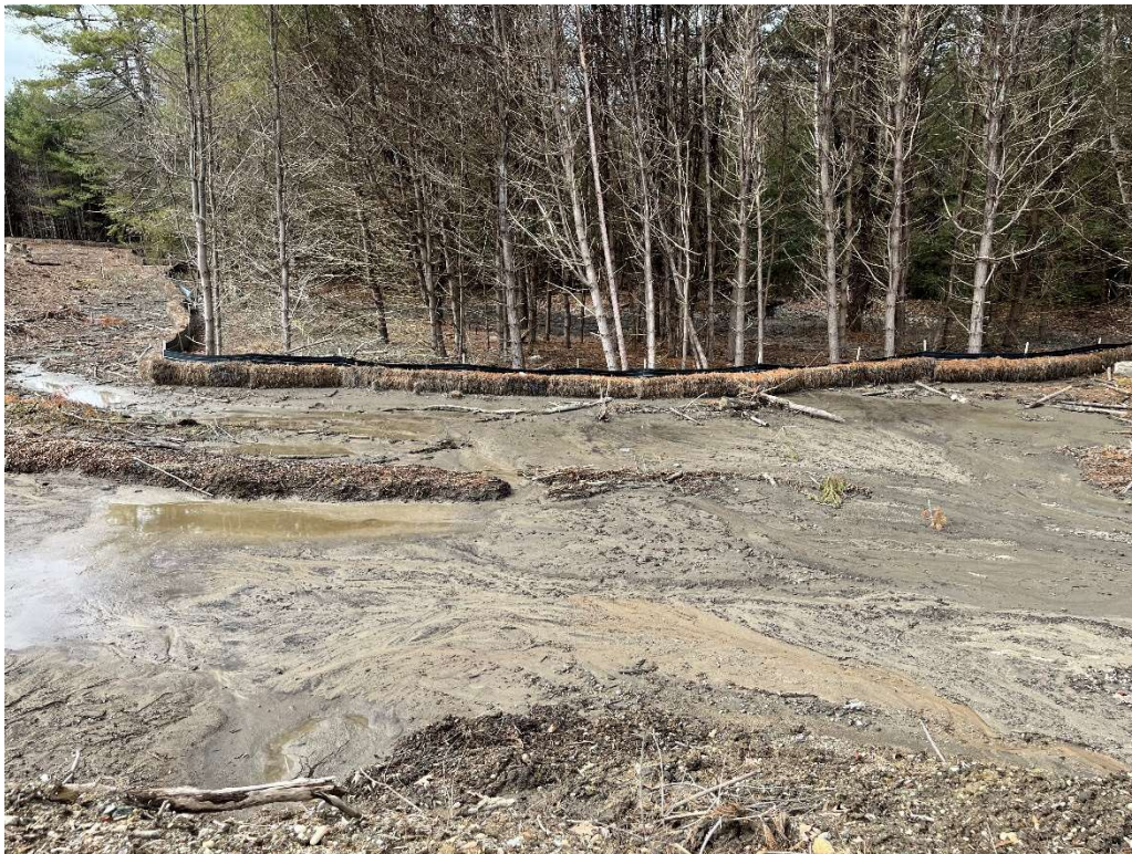
Photo 10 – Silt buildup at southwestern limits of the Site.
