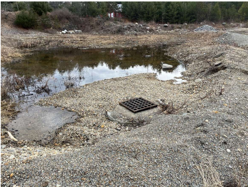
Photo 2 – Temporary stormwater overflow catch basin.
