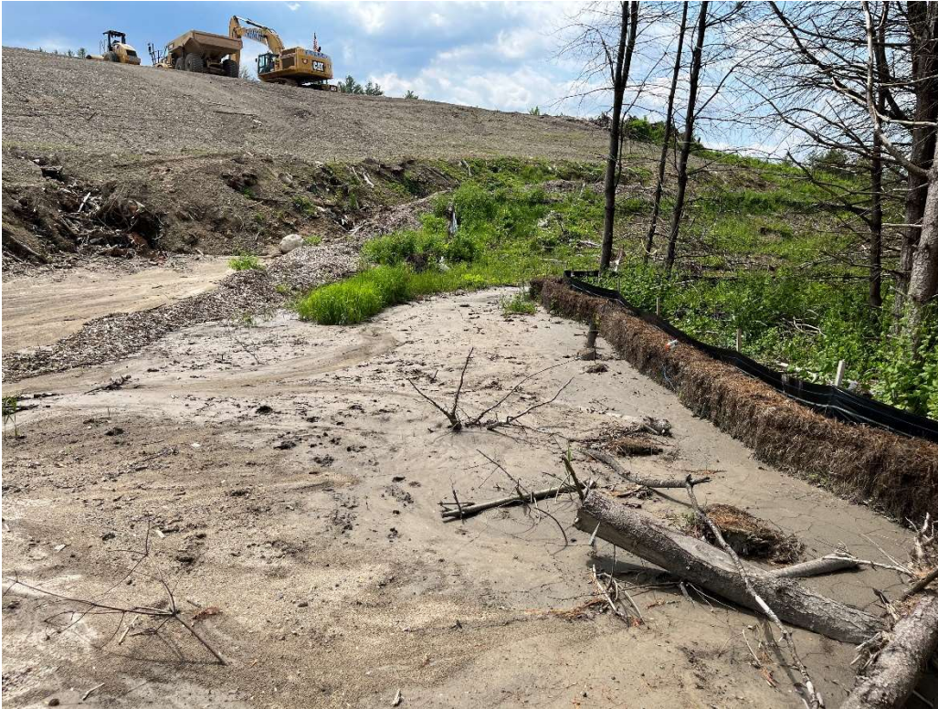
Photo 12 – Silt buildup at southwestern limits of the Site.
