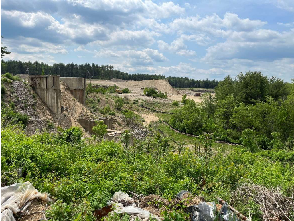
Photo 13 – Existing slope and erosion control at the southern limits of the Site.
