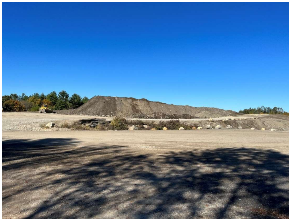
Photo 12 –Material placed and graded at the center of the Site with grading for truck access
