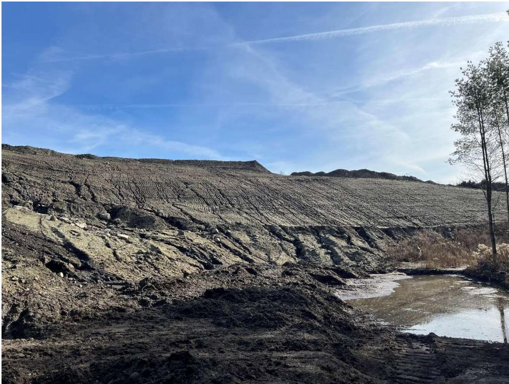
Photo 4 – Southwestern slope with erosion and standing water.
