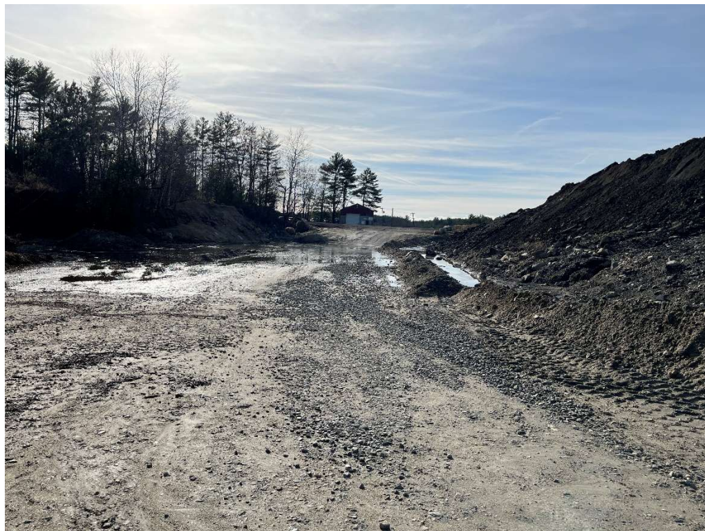
Photo 2 – Eastern slope and damaged access road, looking south.
