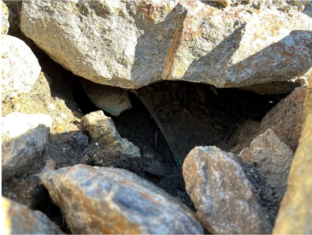
Photo 7 - Broken drainage pipe under added riprap.
