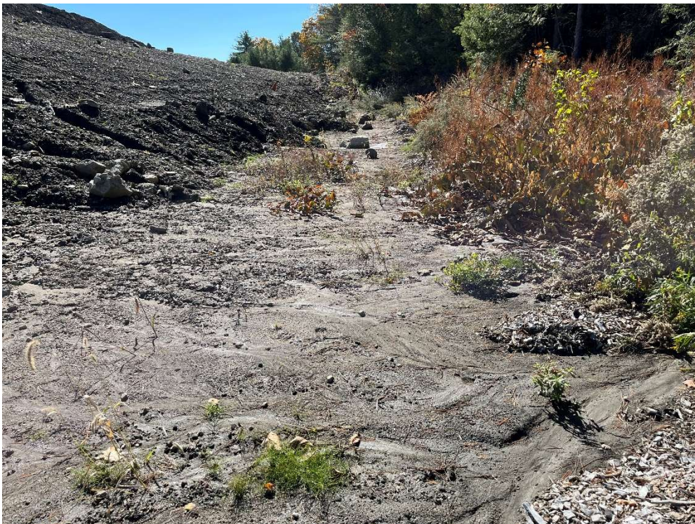
Photo 10 –Erosion control with sediment buildup on the western limits of the Site.
