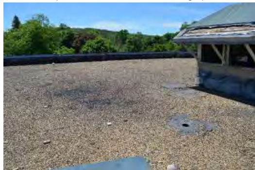
Close up of Southwest Corner of Roof (Wood Framed Penthouse on Right)
