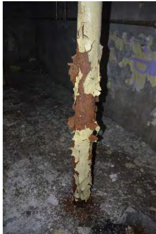
Deteriorated Steel Column in Basement (base)
