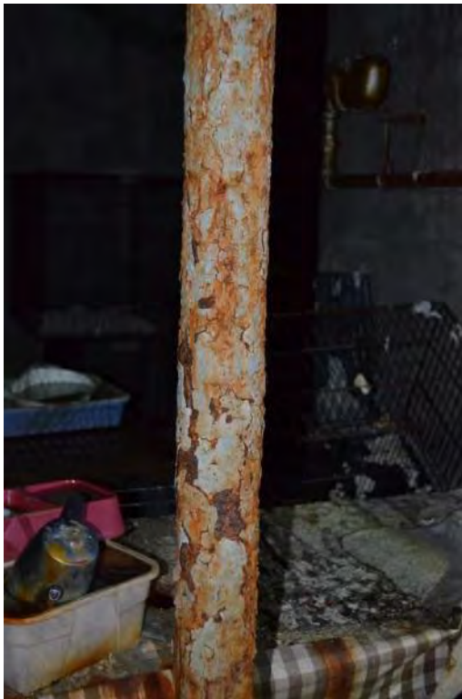
Deteriorated Steel Column in Basement (mid-height)
