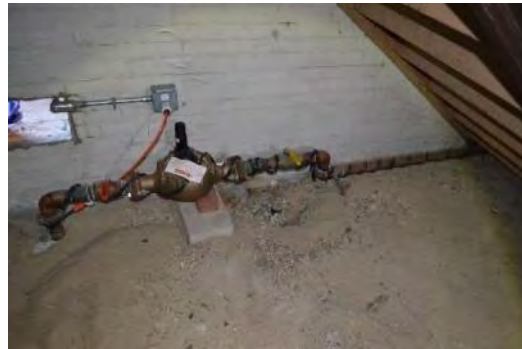
New Pipe and Undermined Slab (North Stair)
