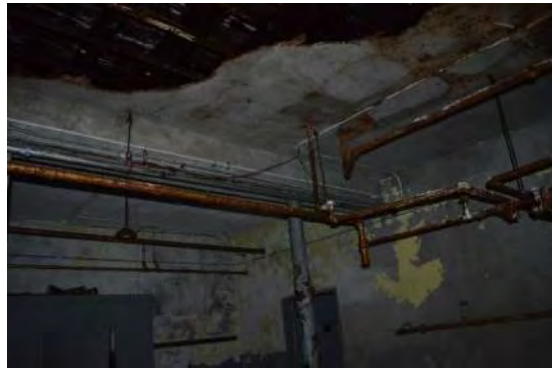
Water Damage in Southwest Corner (Exposed 1 st Floor Framing)
