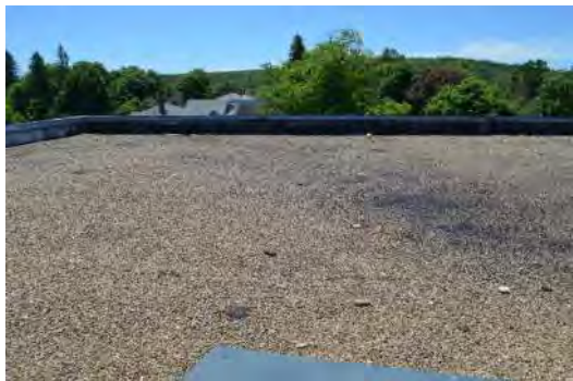
Southwest Corner of Roof (Dark Region is the Location of Breach in Roofing System)
