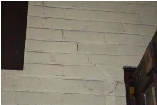
Step Crack Radiating from Door Head
