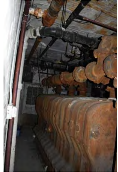
Glimpse into mechanical room
