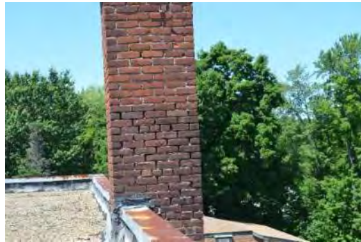
Listing Chimney on North Elevation (deteriorating mortar joints)
