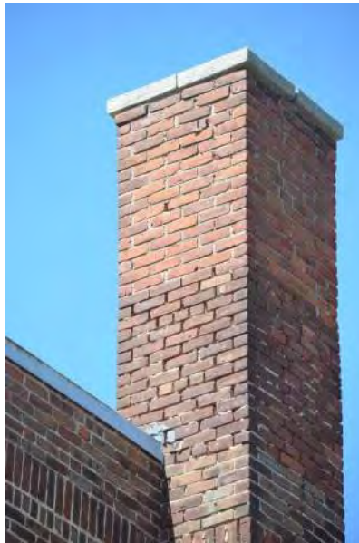
Chimney on North Elevation (deteriorating mortar joints)
