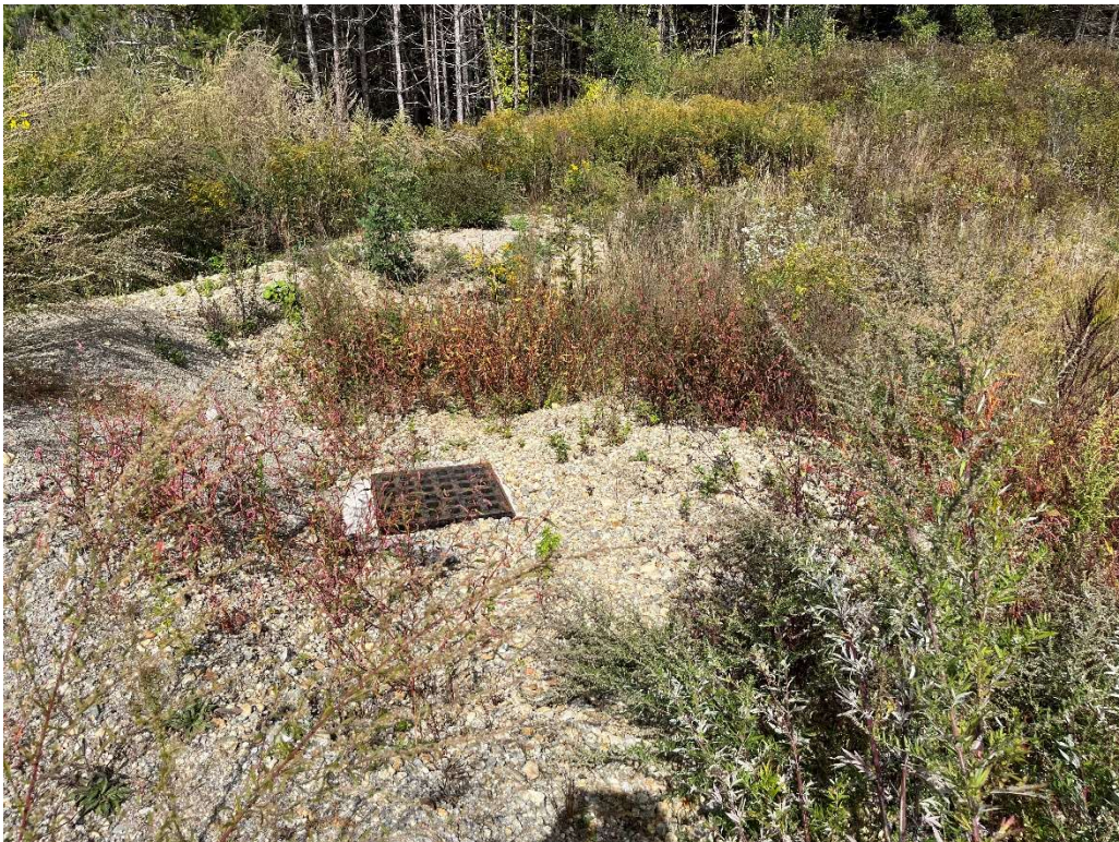
Photo 4 – Temporary stormwater overflow catch basin.
