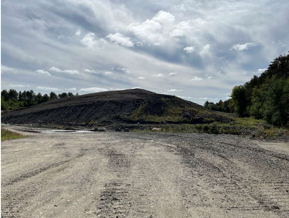
Photo 3 – Northern slope with rill erosion.
