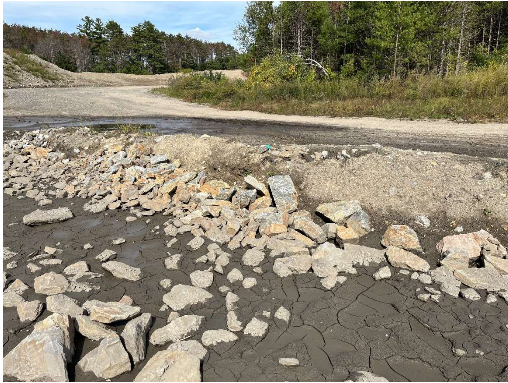
Photo 7 – Location of broken drainage pipe under additional riprap.
