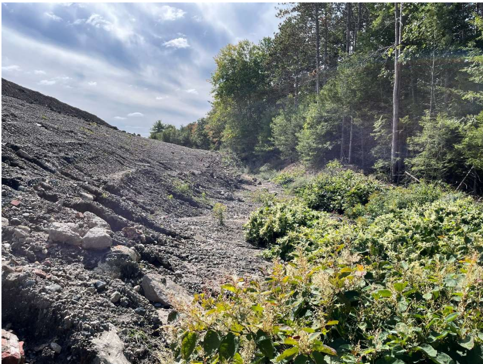
Photo 10 – Representative view of erosion control on the western limits of the Site.
