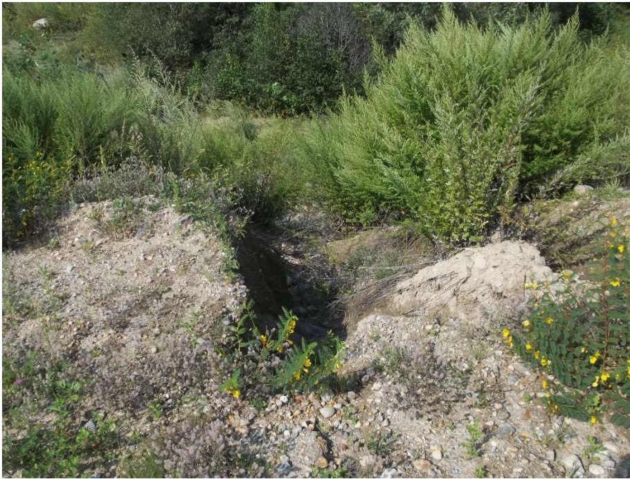
Photo 13 – Erosion in the slope at the southern edge of the landfill.
