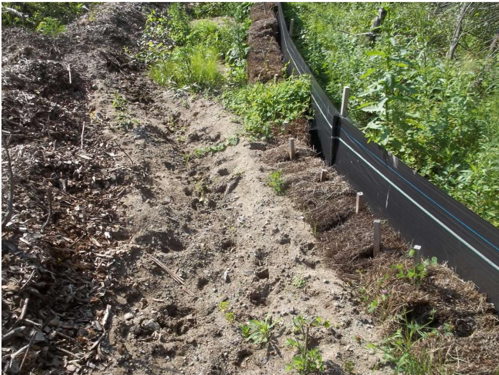
Photo 10 – Erosion control on the western limits of the Site with sediment buildup.
