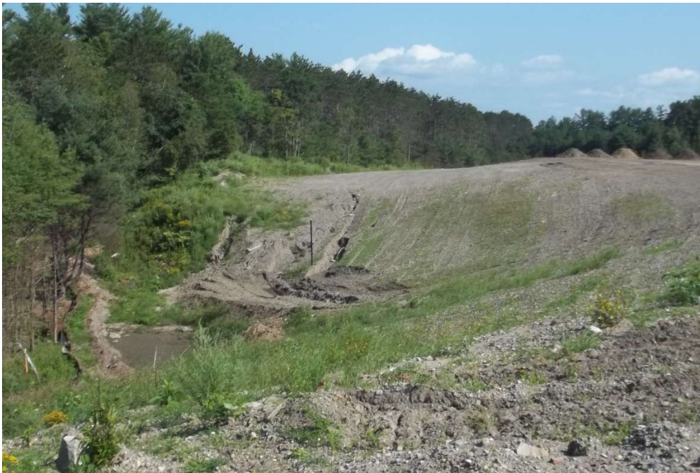
Photo 12 – Western landfill slope including erosion in the area of the monitoring well.
