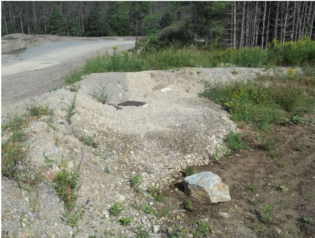
Photo 3 – Temporary stormwater overflow catch basin.
