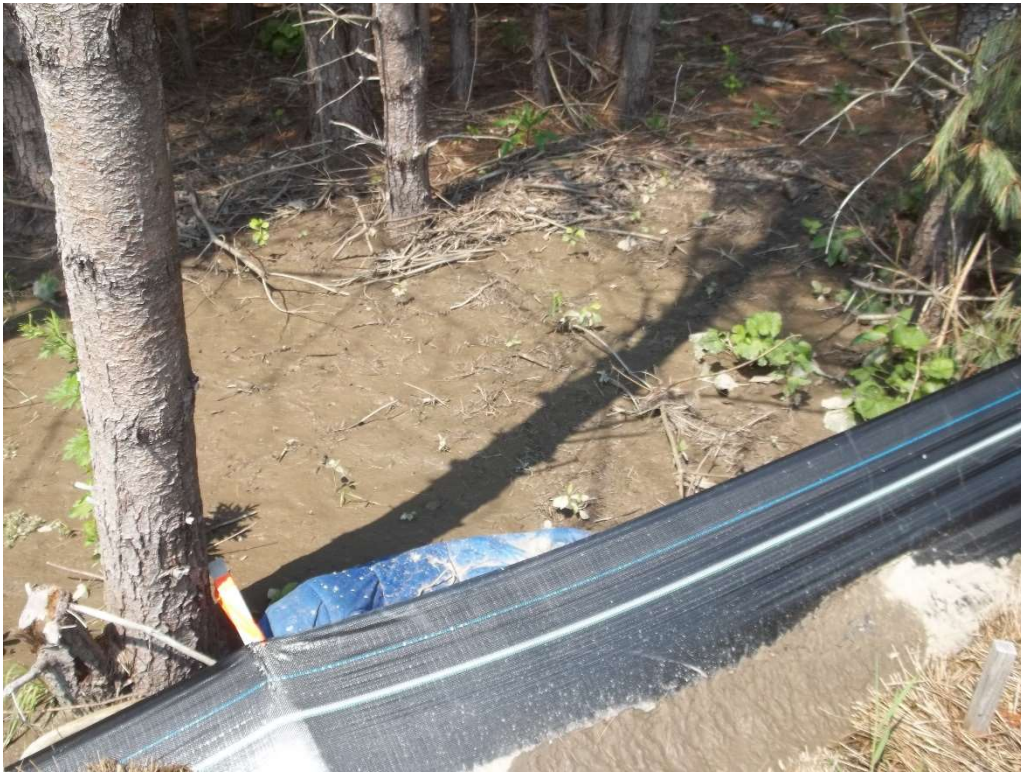
Photo 9 – Sediment overtopping the erosion control on the western limits of the Site.
