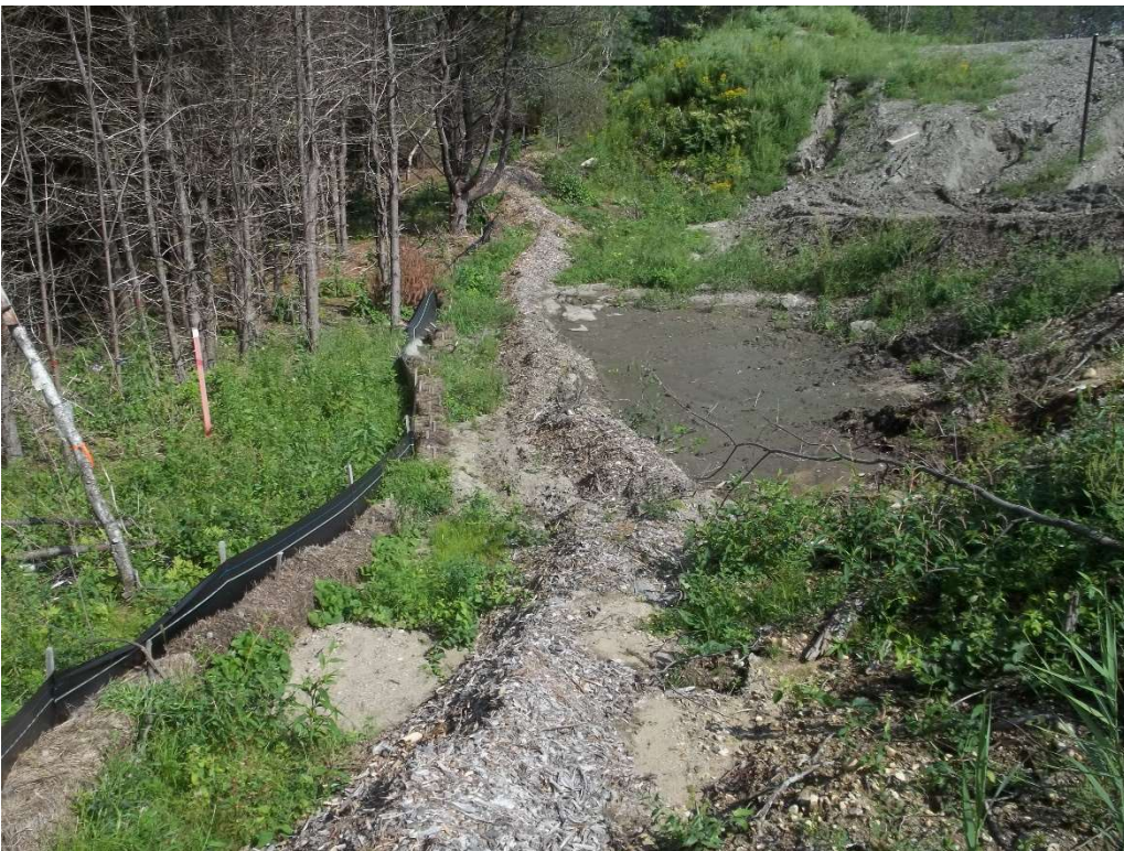
Photo 8 - Sediment buildup and damaged erosion control on the western limits of the Site.
