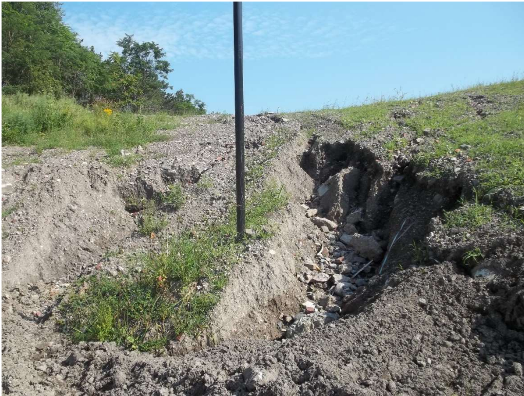
Photo 11 – Erosion in the subgrade slope adjacent to a monitoring well.
