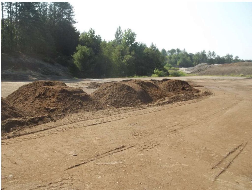
Photo 2 – Material placed to be shaped on the northern section of the site.
