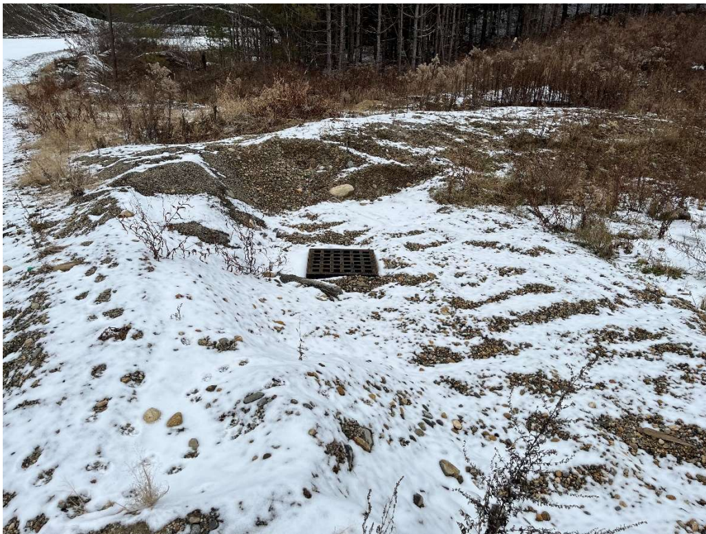
Photo 2 – Temporary stormwater overflow catch basin.
