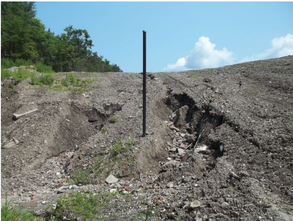
Photo 10 – Erosion in the subgrade slope adjacent to a monitoring well.
