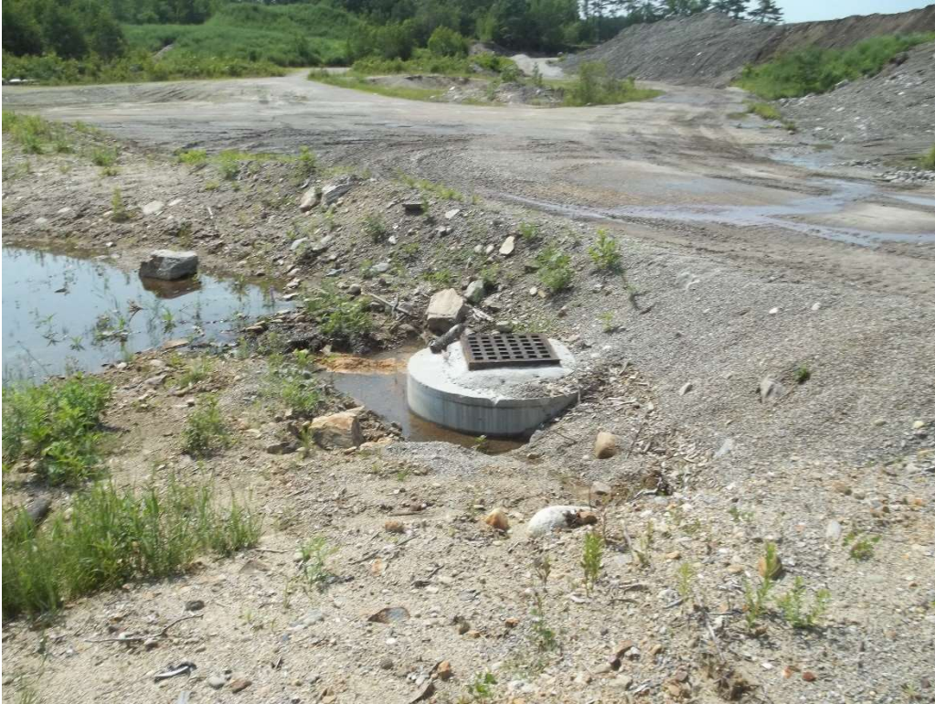
Photo 3 – Temporary stormwater overflow catch basin.
