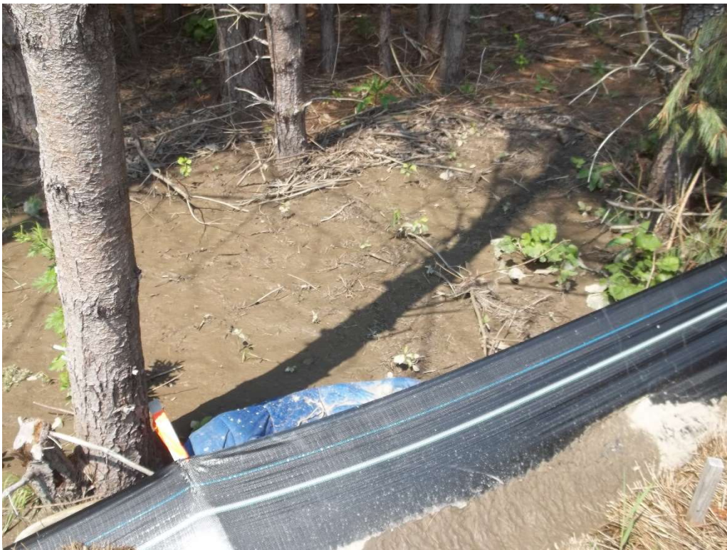
Photo 8 – Sediment overtopping the erosion control on the western limits of the Site.
