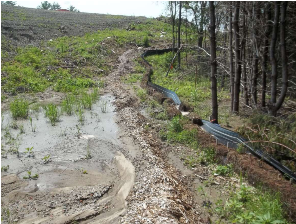
Photo 7 – Sediment overtopping the erosion control on the western limits of the Site.
