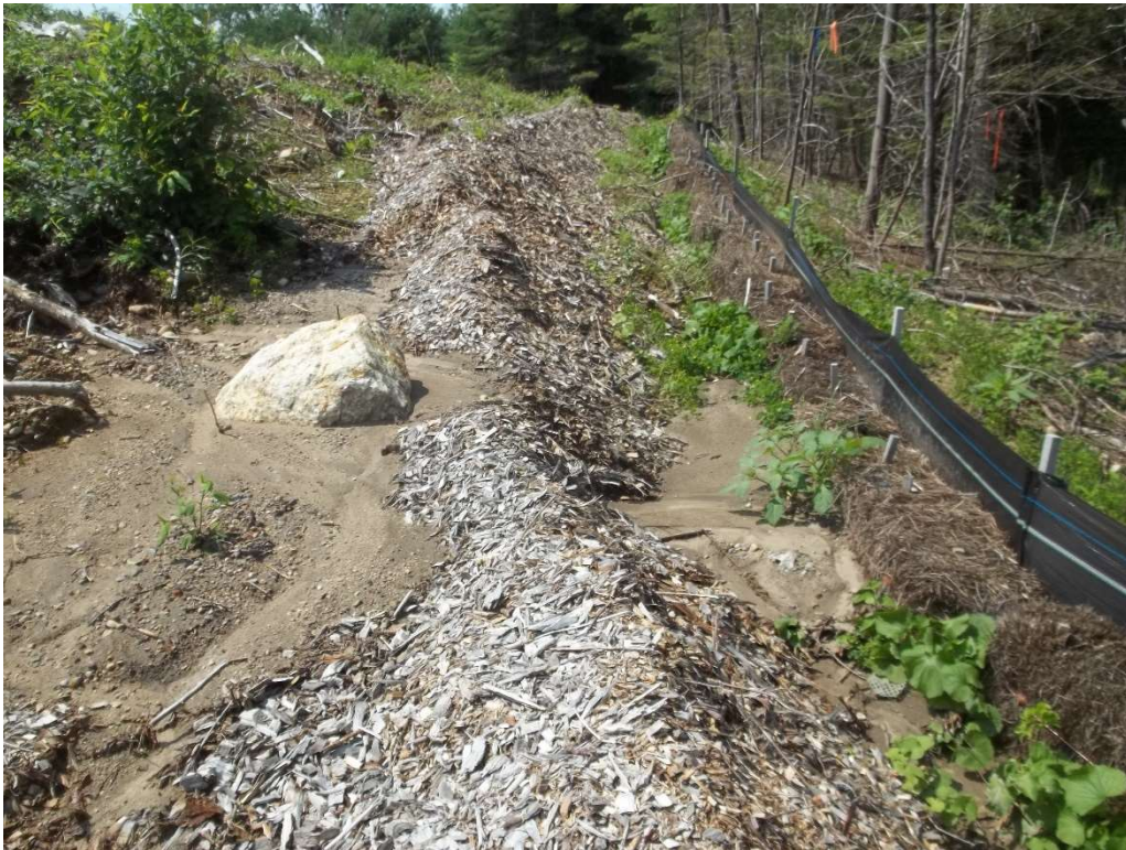
Photo 9 – Erosion control on the western limits of the Site with sediment buildup.
