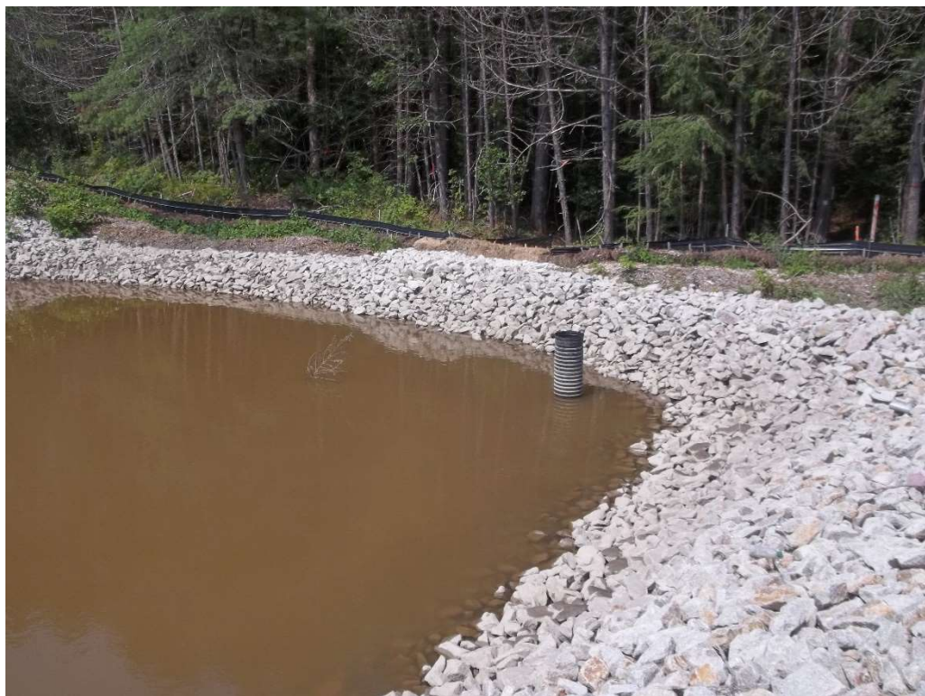
Photo 6 - Temporary rip rap settling area with sediment and standing water.
