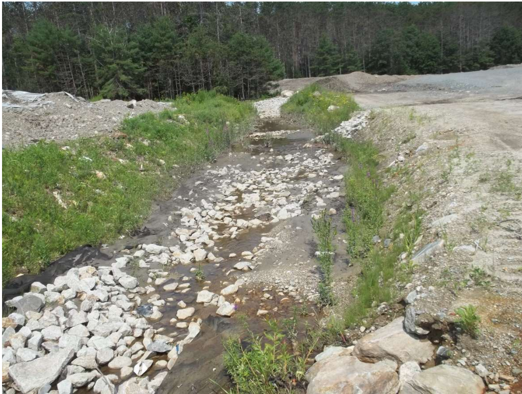
Photo 5 - Swale and check dams between temporary stormwater basin and temporary rip rap settling area.
