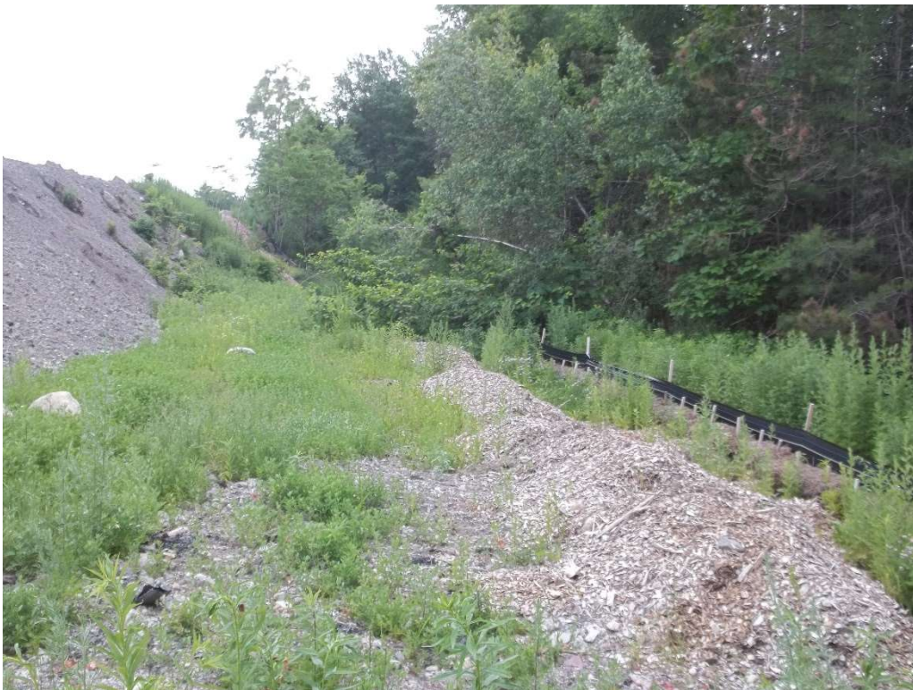
Photo 5 - Representative view of erosion control on the western limits of the Site.
