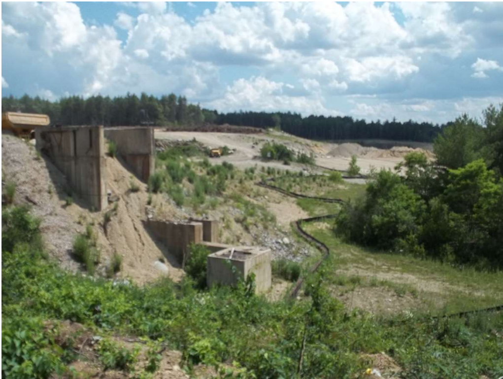
Photo 6 – Existing slope and erosion control at the southern limits of the Site.
