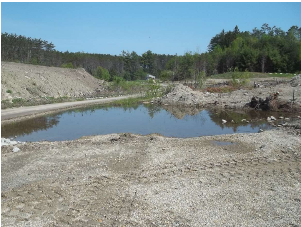
Photo 2 – Temporary Stormwater Basin. 4' high berm with rip rap overflow not yet constructed.
