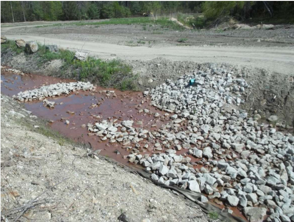
Photo 3 - Swale and check dams between temporary stormwater basin and temporary rip rap settling area.
