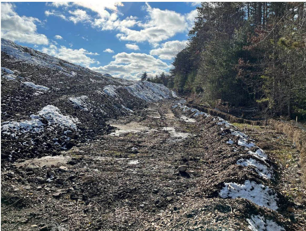
Photo 8 – Representative view of erosion control on the western limits of the Site.
