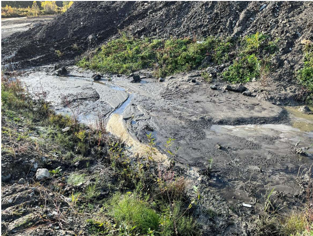
Photo 5 – Sediment built up in swale between temporary stormwater basin and temporary rip rap settling area.
