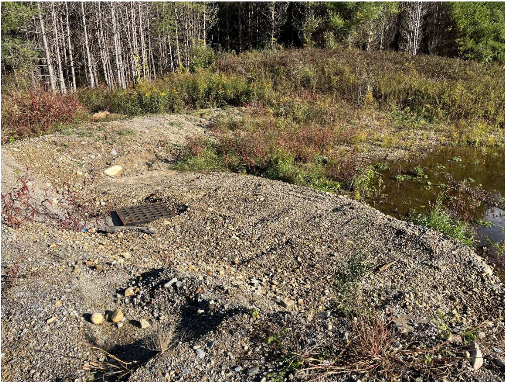
Photo 3 – Temporary stormwater overflow catch basin.
