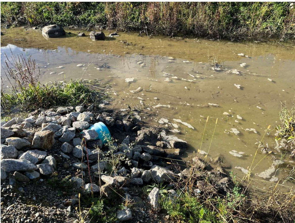
Photo 4 – Stormwater culvert under access road, sediment and standing water in swale.
