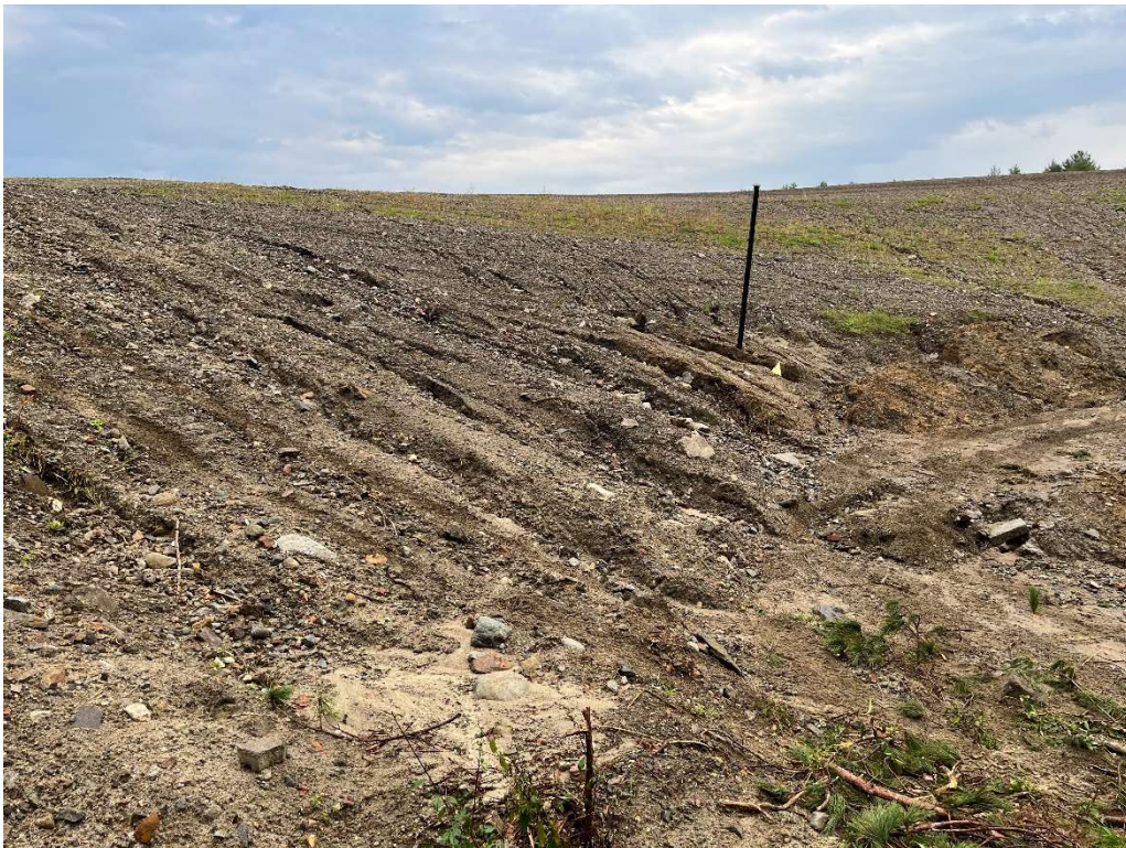
Photo 10 – Repairs and continued erosion in the subgrade slope adjacent to a monitoring well.
