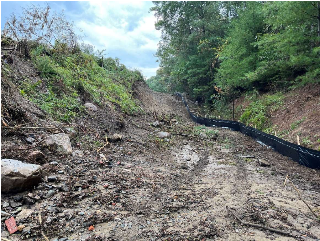
Photo 9 – Vegetation clearing at the western limits of the Site for erosion control replacement.
