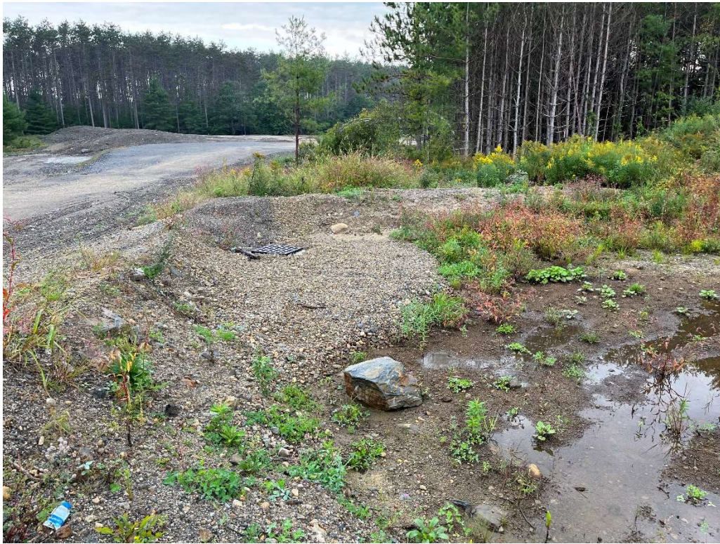
Photo 3 – Temporary stormwater overflow catch basin.
