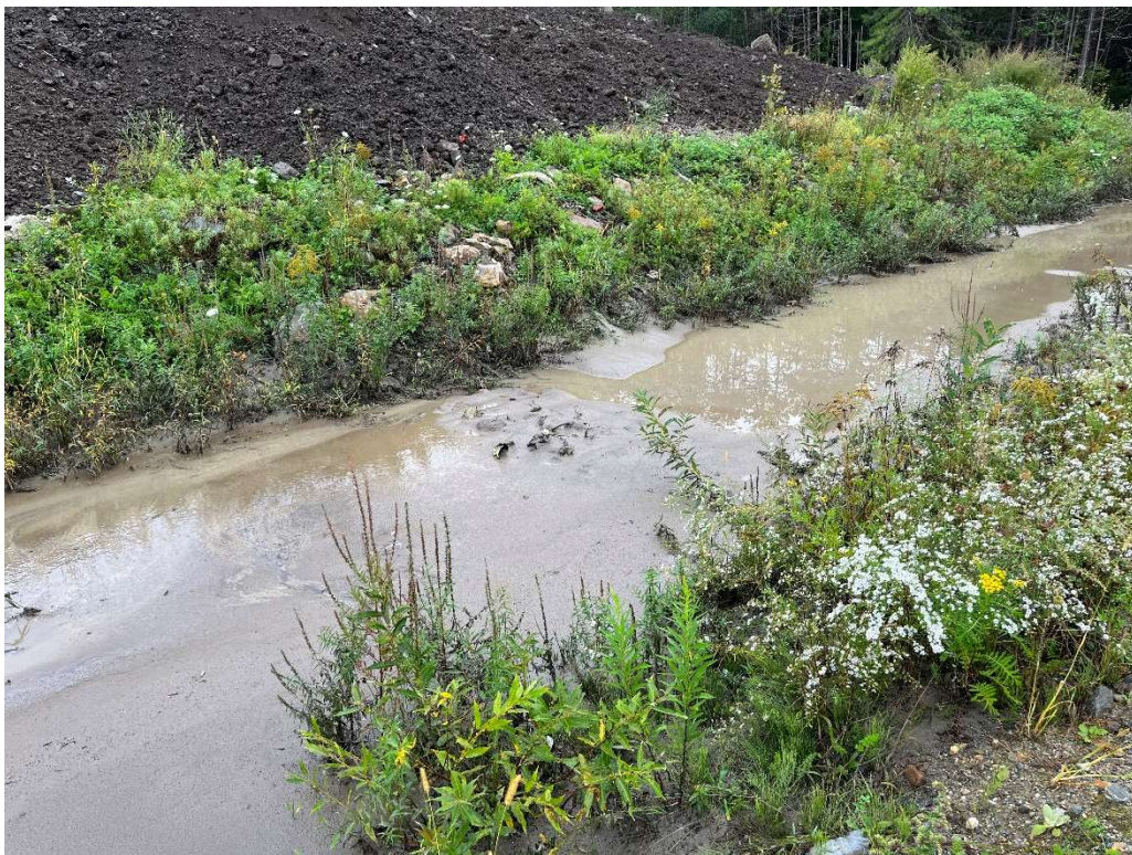
Photo 6 - Check dam and sediment buildup between temporary stormwater basin and temporary rip rap settling area.
